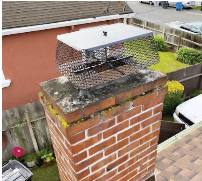
Healthy Home Connect tackles many home repairs that can benefit health and energy use such as properly venting a chimney. PHOTO COURTESY HEALTHY HOME CONNECT
