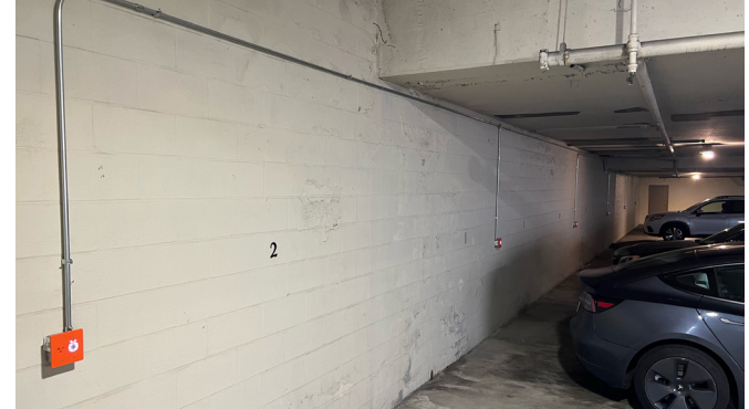
Smart charger outlets installed in garage
