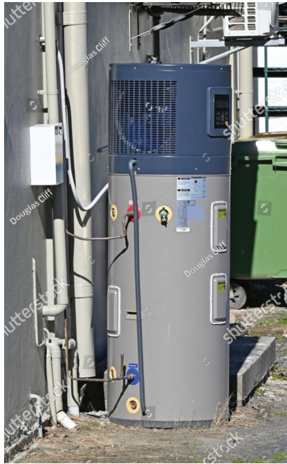
Heat pump water heater
